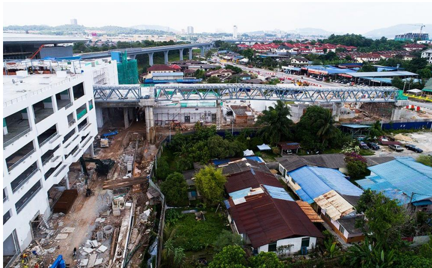
Figure 1: MRT Station Being Built Alongside the Remaining Village of Kampung Bukit Dukung at Jalan Cheras, Kajang in 2017
