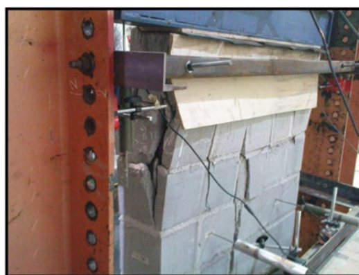
FIGURE 16. Local crushing on masonry
