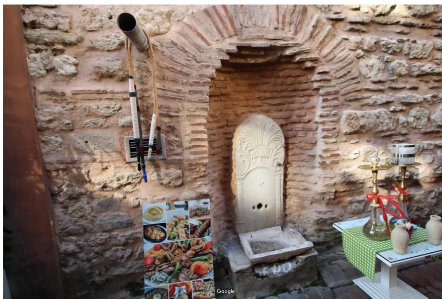
Figure 4: Missing Spout on the Cevri Kalfa Sibyan Mektebi Cesmesi. Note the Appropriated Niche. (Source: map.google.com)
