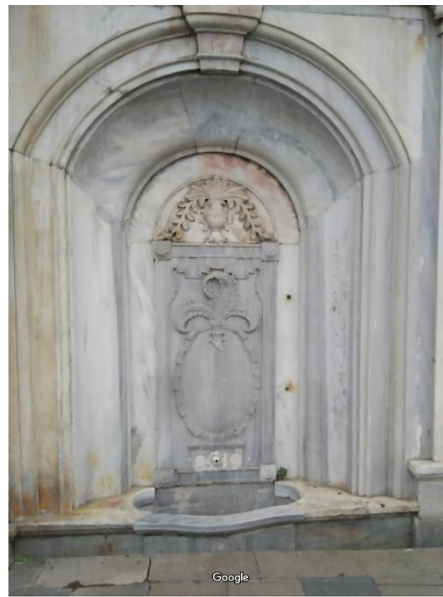
Figure 3: Missing Spout on the Cevri Kalfa Cesmesi. Note the Untouched Niche. (Source: map.google.com)
