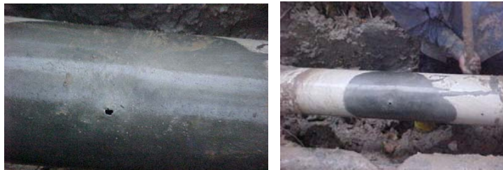
Figure 9 Surface condition of API 5LX42 pipe
