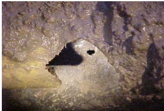
Figure 13 On-site condition of damaged PE due to gas jet from API 5L X42 pipe
