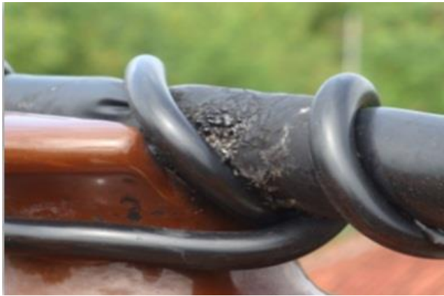
Figure 1 Sheath degradation of AAAC-S
