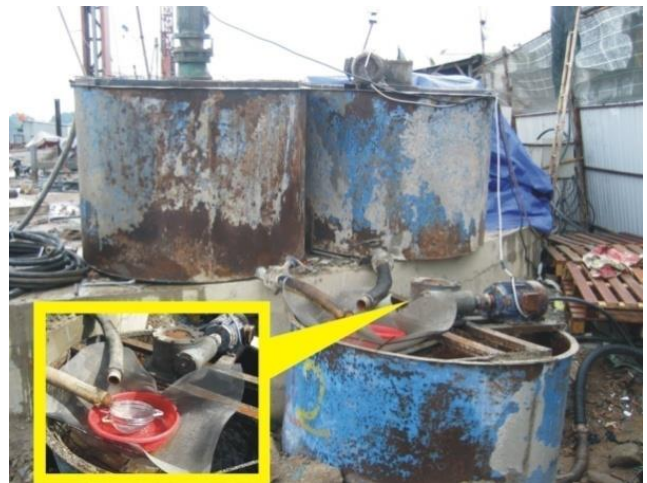
Figure 5 A cement slurry mixing system
