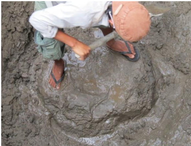
Figure 9 0.8 m diameter of the trial soilcrete column No. 1 excavated after 7-day construction
