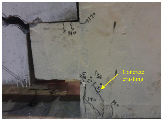
Figure 8 Crushing of corbel support
