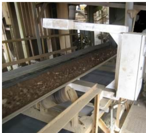
Figure 2 Installation of SM moisture analyzer belt conveyor in nickel ore mining
