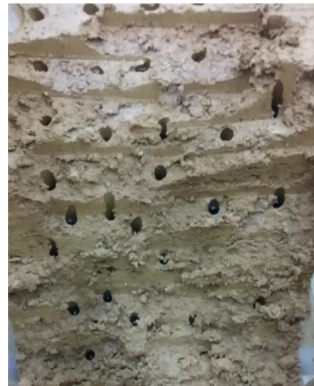
Figure 4 Infiltrating water hold in the burrow hole
