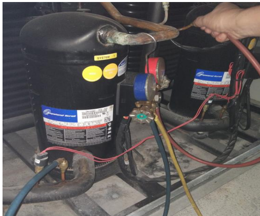
Figure 11 The maintenance checking of compressor
