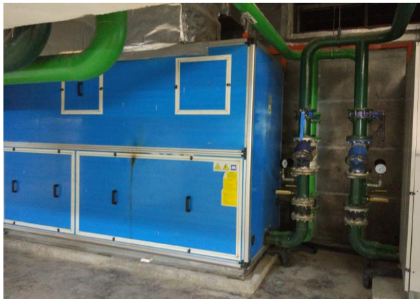
Figure 1 A WCPU placed in AHU room
